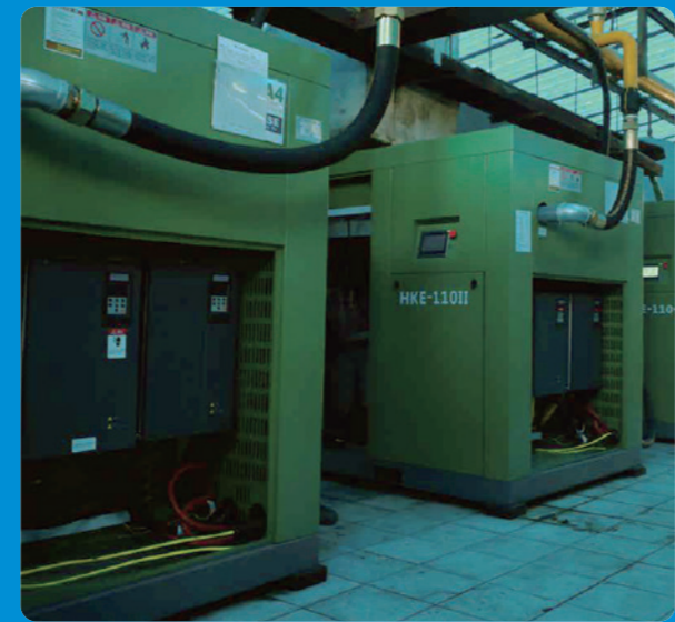
Automatic control system of air compression station
